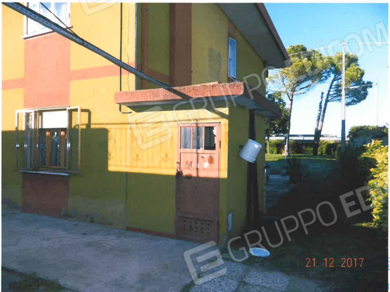
LOTTO 1 – Centrale termica (particella 32, sub. 4) – piano terra
